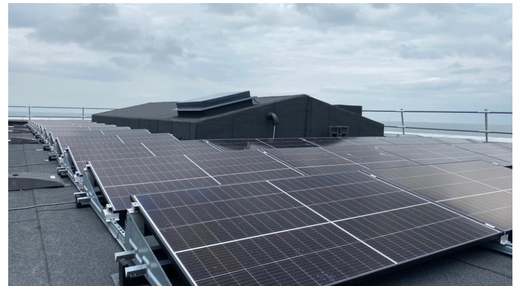
Figure 3.1.1: Rooftop solar PV
