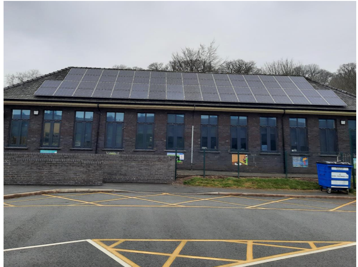
Figure 4.1.1: Ysgol Betws Gwerfil Goch solar PV array, Corwen, Denbighshire
