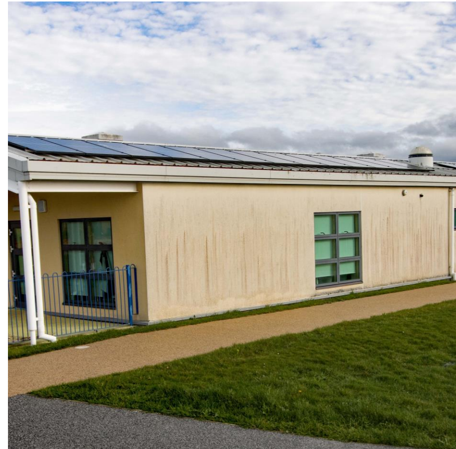
Figure 3.2.1: Ysgol Tir Morfa rooftop solar PV, Rhyl, Denbighshire
